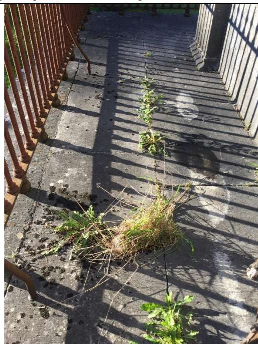
Weeds and vegetation growth between paving
