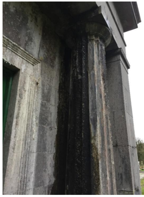
Water saturation to external walls
