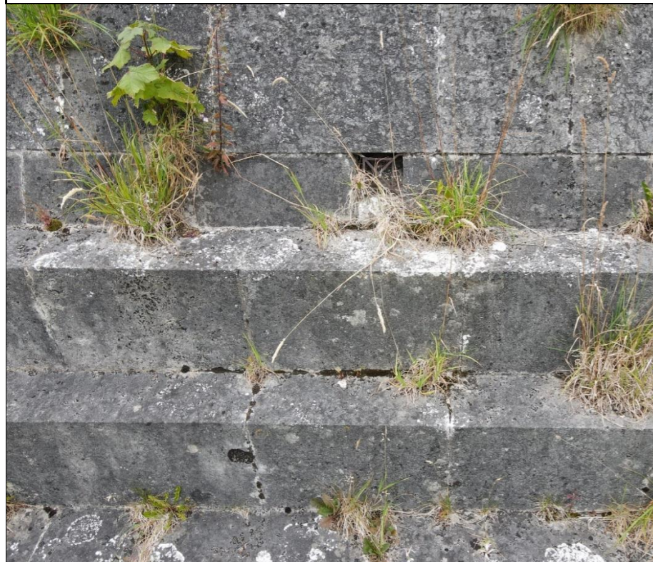
Close up of vegetation growth and vent detail
