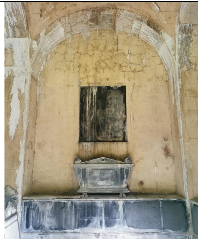
Interior of mausoleum showing extensive water ingress
