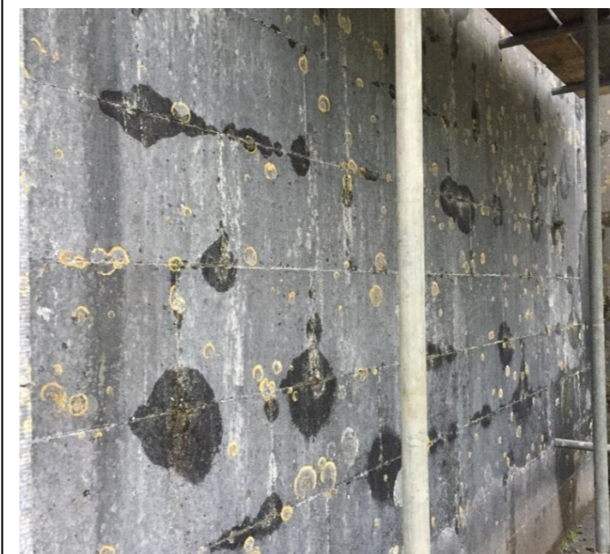
Water saturation to external walls
