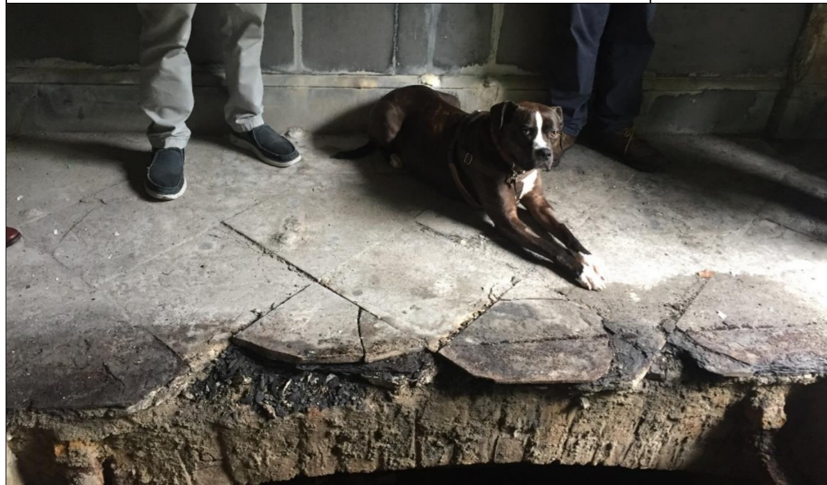
Chequered stone floor detail with damage to floor edging
