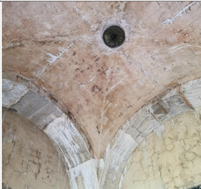
Interior of mausoleum showing extensive water ingress
