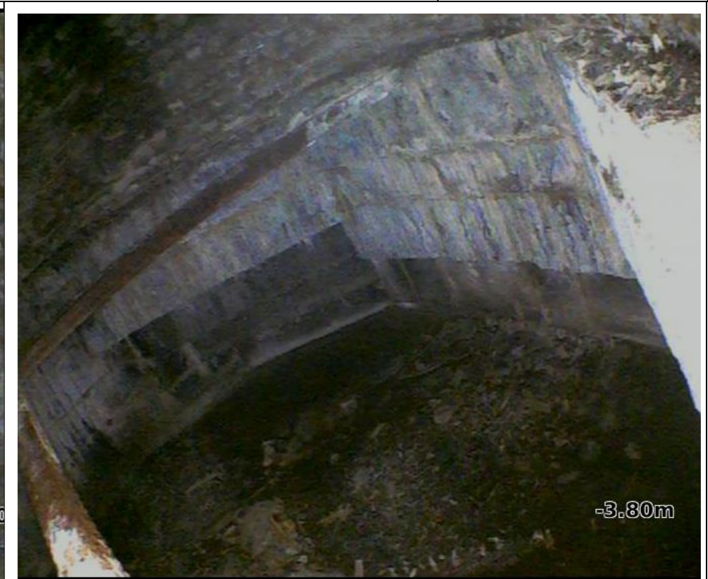
Interior view showing pooled water to corners above groin vault
