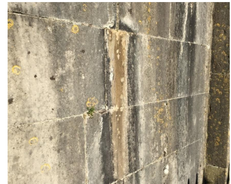
Staining and water damage to external façade.
