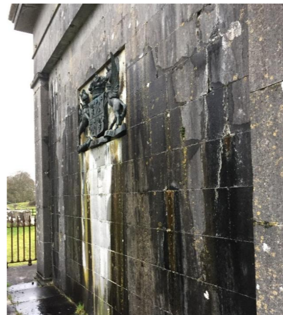
Water saturation to external walls
