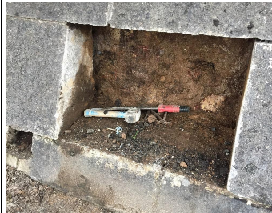
Gaps behind stonework allowing water ingress
