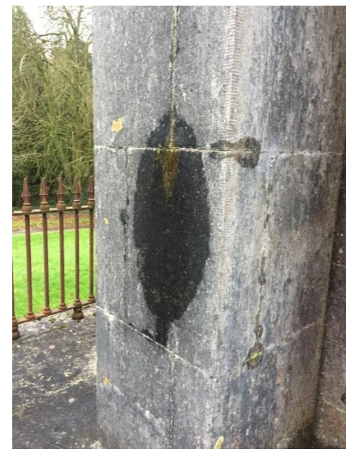
Water saturation to external walls
