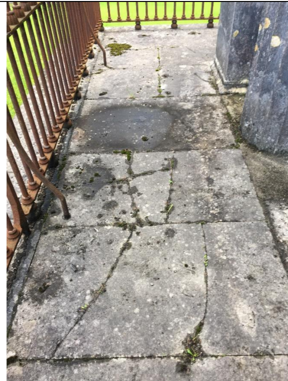
View of cracked paving slabs to north-east side
